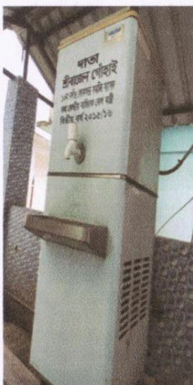
Cold water unit
