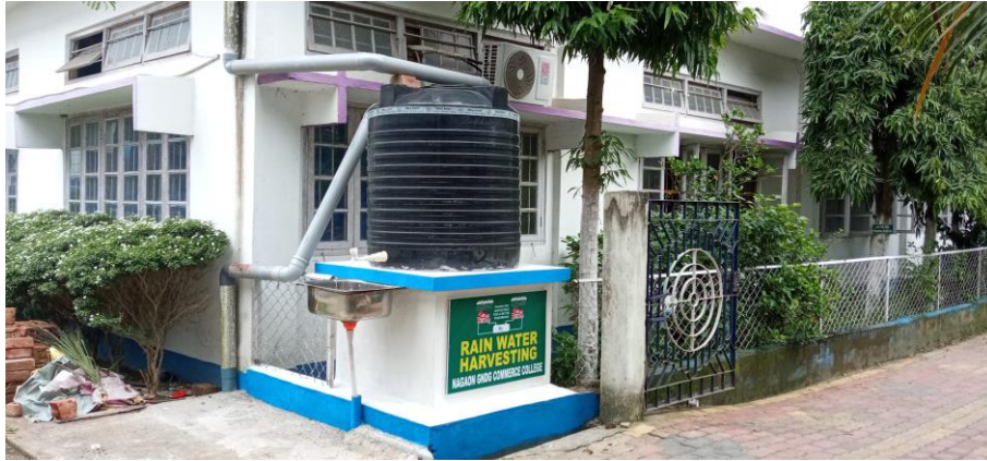
Rain water Harvesting
