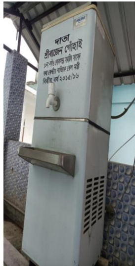
Cold water unit
